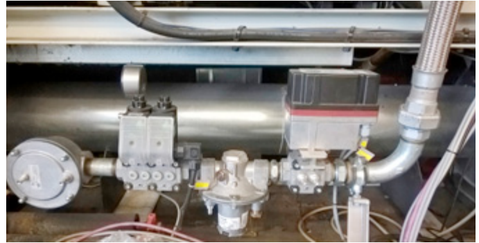
CHP for generating electricity and heat
